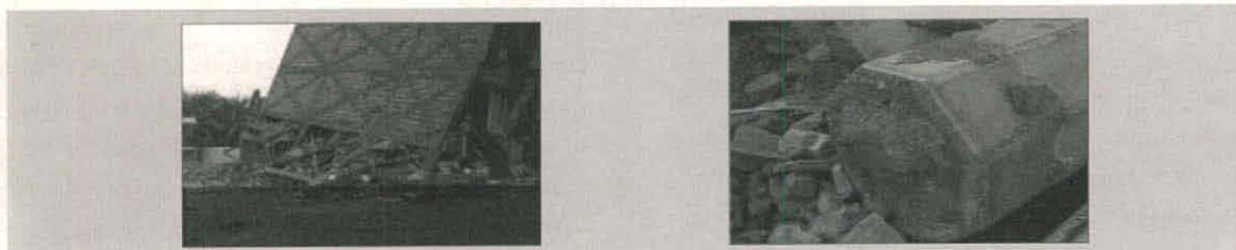
Figure 5- Use of steel below the standard amounts in concrete structures, lack of connection of columns with the foundation, and omission of wind brace in steel structure and the formation of soft storey
