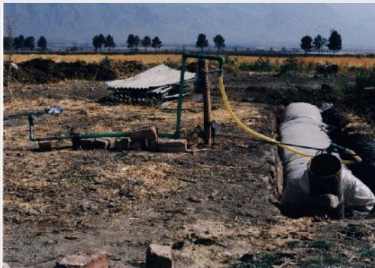
Figure 2. Installed polyethylene biogas plant.
